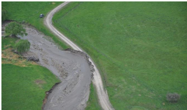
Erosion into a farm road along the Upper Murray River, NE Victoria, after the 2010 floods; photo by Ian Rutherford.
